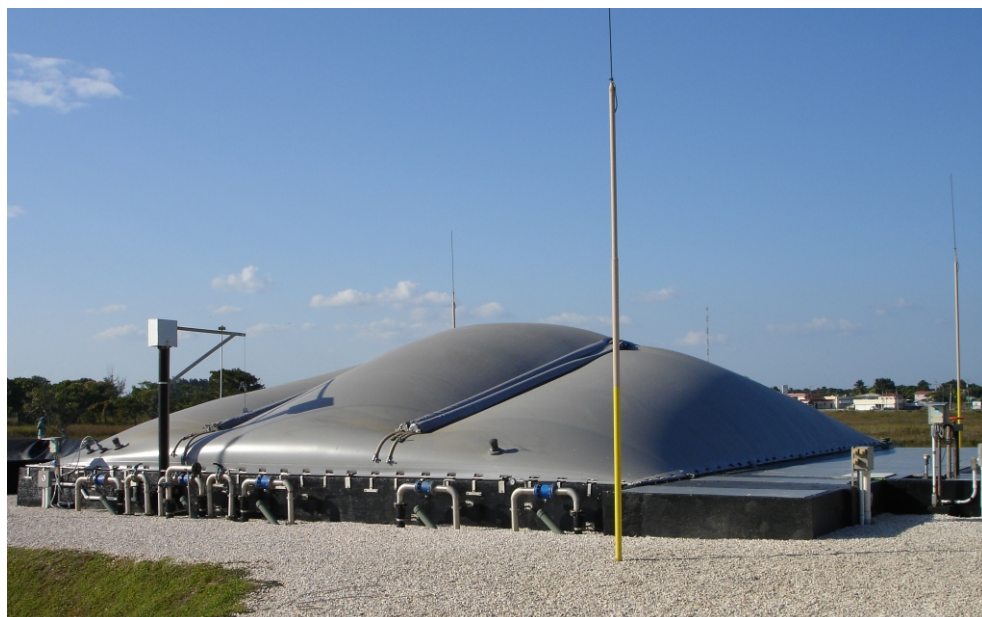
BIOLAK ® GAS Liquid plant for soft drinks production of approx. 1,200 m 3 /d, 2,450 kg COD/d
